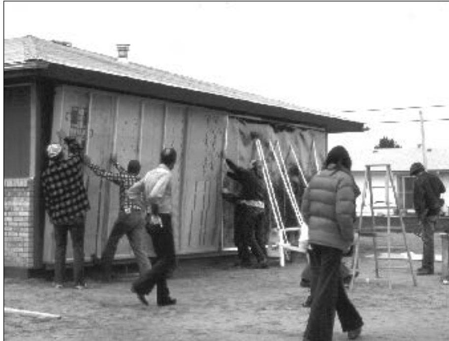
Homemade air collectors are retrofitted onto an existing home as a neighborhood project.
